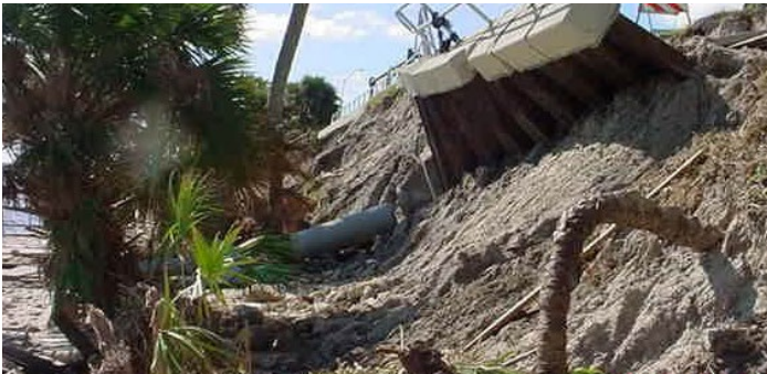
PROBLEM Damaged side slopes leave highway vulnerable to falling into river
