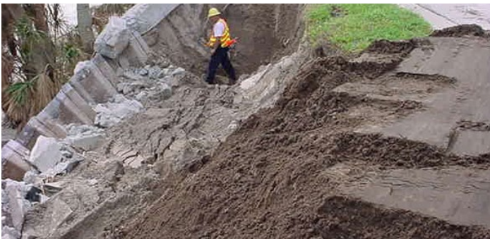
INSTALLATION Assessment of the damage and project solution after hurricane
