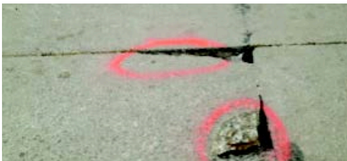
PROBLEM 50 years of use cause major drainage issues on US 10E
